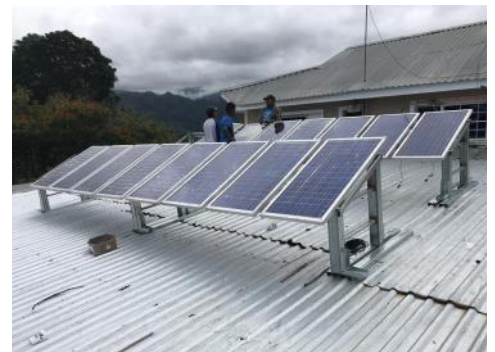
Solar Panels on Boys' House
